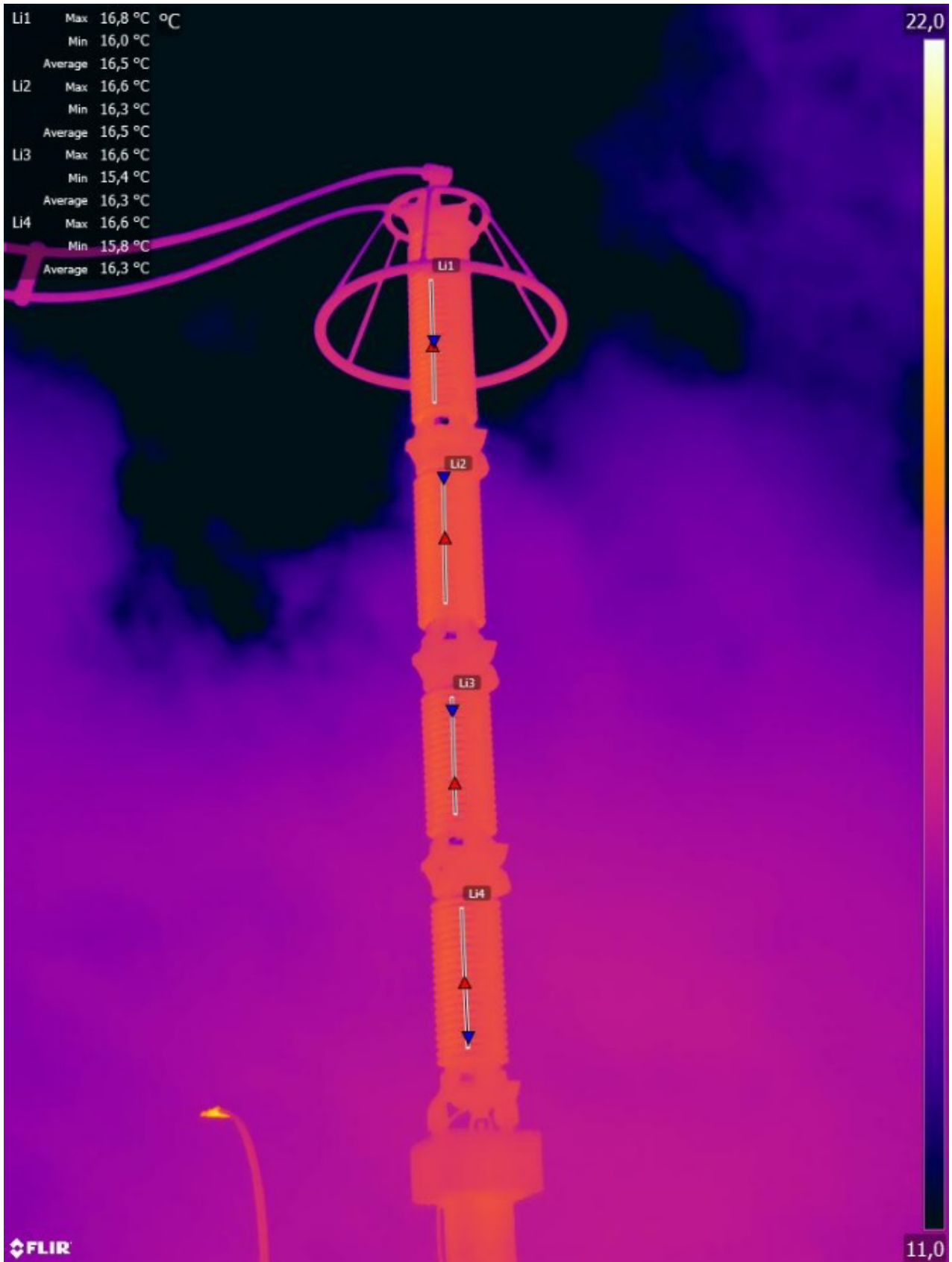
Figure 17 - A manually processed image of an arrester in which the main-axis of each section was selected.
